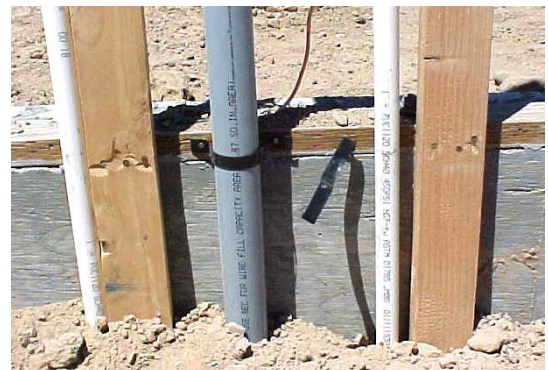
Figure 4 Conduit Support Strap Attached To Sill Plate
